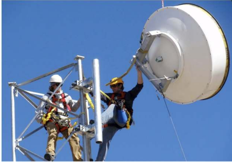
Figure 12 Justin and Jason Davis of Skywerx installing microwave near Crestone, CO. Photo by Skywerx
