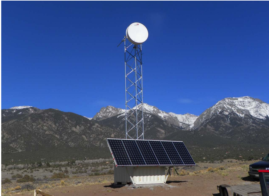
Figure 1 Microwave middle mile near Crestone, CO. Photo by Justin Davis
