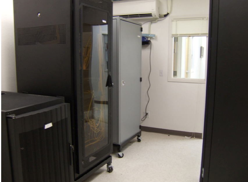
Figure 14 Carrier neutral location for City of Cortez, CO which as a result enjoys 3 middle mile providers and 4 last mile providers. Photo by Corey Bryndal
