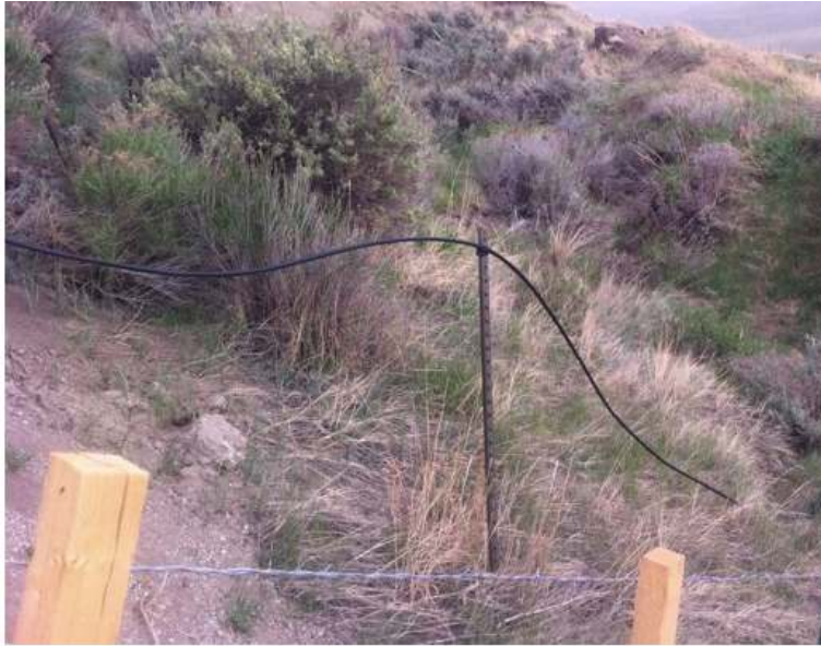
Figure 7 Spring 2012: fiber optic cable (black line above fence line) allegedly owned by telephone company with market cap of $26 billion along US 50 between Montrose and Gunnison, CO exposed by landslide. Note how rancher has installed new fence where the telephone company leaves fiber optic cable (and livelihoods of Gunnison county residents) open to elements. Cattle are more valuable than cable? Photo by Corey Bryndal
